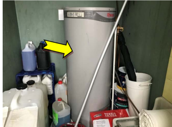
Photo 2. Interior, female toilets, store cupboard, hot water heater – suspected SMF internal insulation material.
