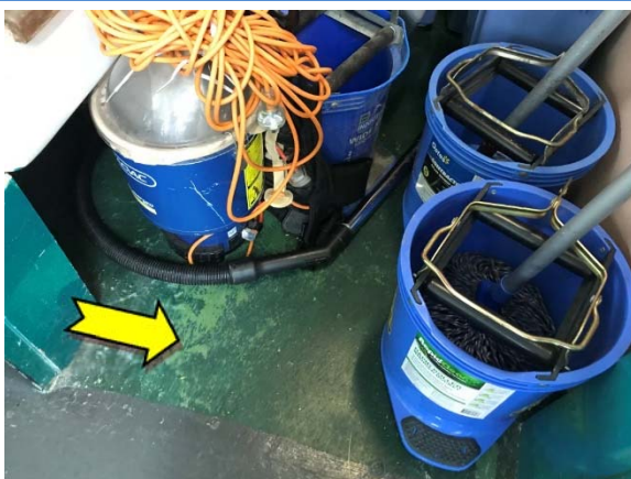
Photo 5. Interior, male toilets, store cupboard, floor – suspected lead-containing dark green upper and light green lower coloured paint systems.
