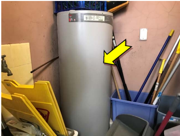
Photo 3. Interior, men's toilets, store cupboard, hot water heater – suspected SMF internal insulation material.
