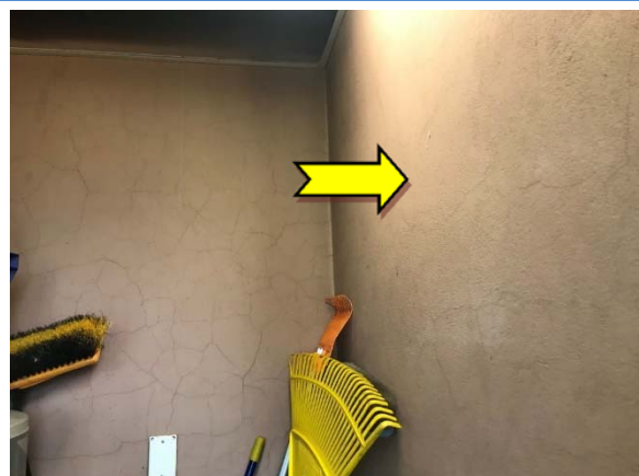
Photo 6. Interior, male toilets, store cupboard, walls – suspected lead-containing pink upper paint systems.
