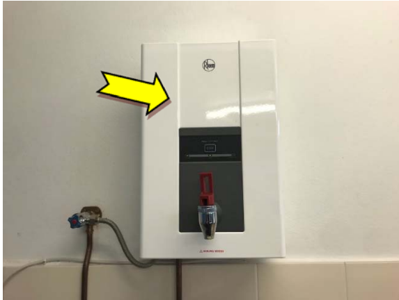
Photo 1. Interior, office, hot water boiler – suspected SMF internal insulation material.
